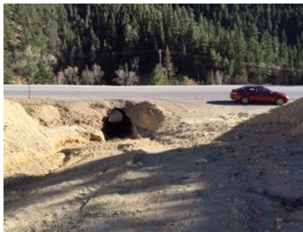
Photos of debris flow hazard area on mile marker 8 on Hwy 38 near Red River (Brislawn)
